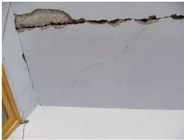
楼板通长裂缝
